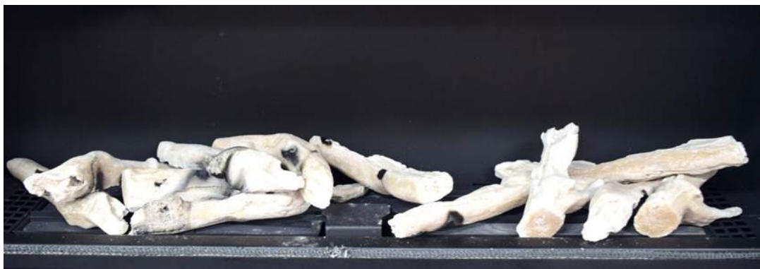
Incorrect Media Installation
