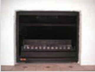
Existing Jetmaster wood fire
